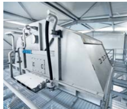
A new disc filter (below) was also part of the ANDRITZ delivery. ▼
